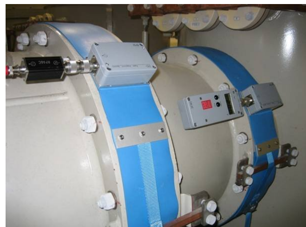
External flange sensor EFS1 (provisionally installed)
