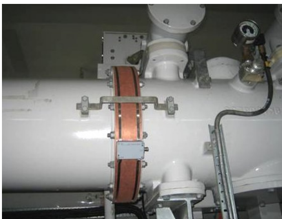
External flange sensor EFS1 (permanently installed)
