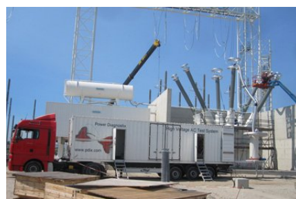
Fig. 16: On-site high voltage test on 500 MVA current limiting reactors
