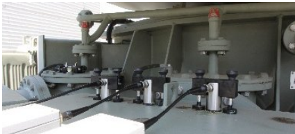
Fig. 20: Online acoustic detection on a transformer oil bushing
