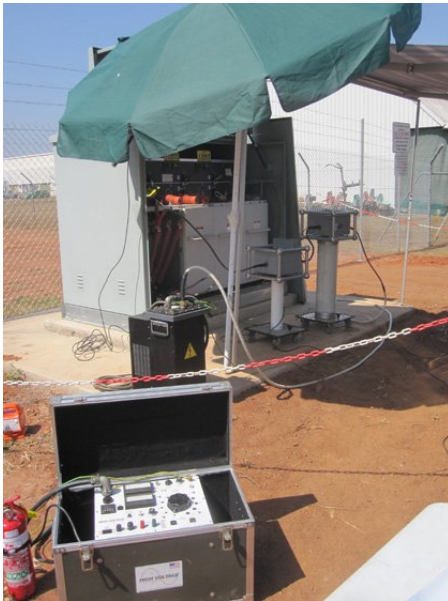
Fig. 15: On-site PD and TD test on medium voltage cables using VLF (0.1 Hz)
