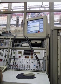
HV control room
