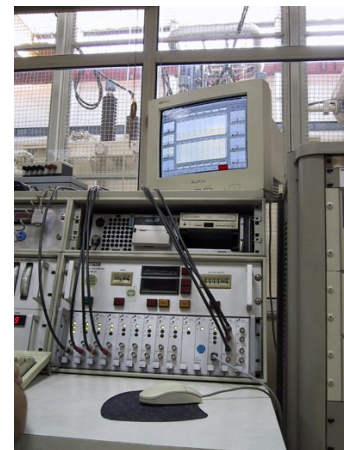
ICMsys8 installed in a control room
