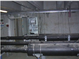
400 kV cable joints
